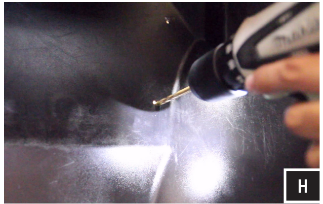
H. Using a 1/4 drill bit, drill holes for mounting of the enclosure.
